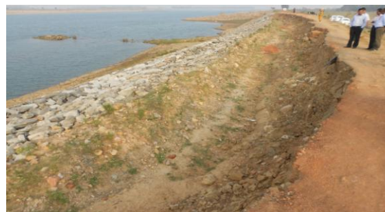
Fig.No.5. Subsidence of Right Embankment
