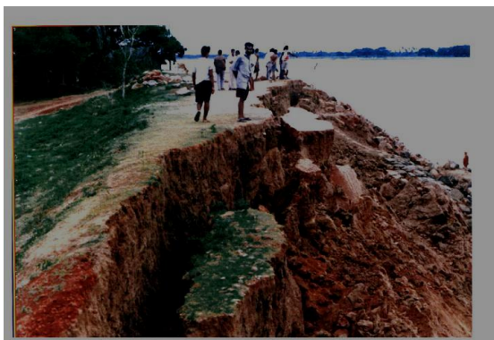
Fig.No. 4. Embankment Subsidence during 2008
